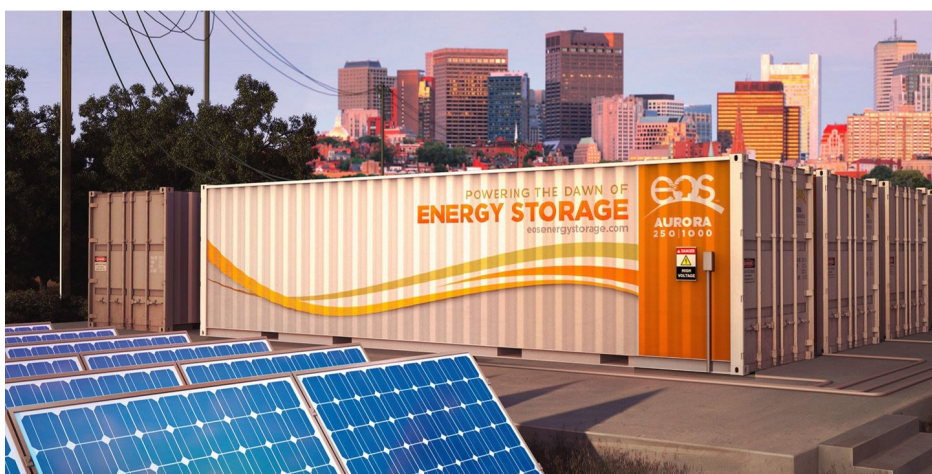
Zinc hybrid cathode battery being installed at Pacific Gas and Electric's San Ramon Advanced Technology Services testing facility. Source: Eos Energy Storage
